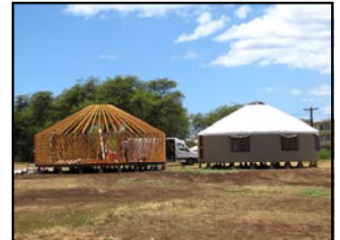
Each of these structures measures 30 feet in diameter and can comfortably seat 25 adults or 30 children. The sky dome at the top center can open up to let out warm air as it rises.
